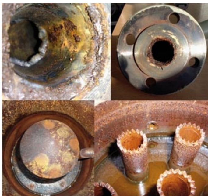
Fig. 4. Corrosion of carbon capture plant elements
