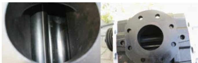
Fig. 9. Blower rotor (left) and compression module (right) after repairs
